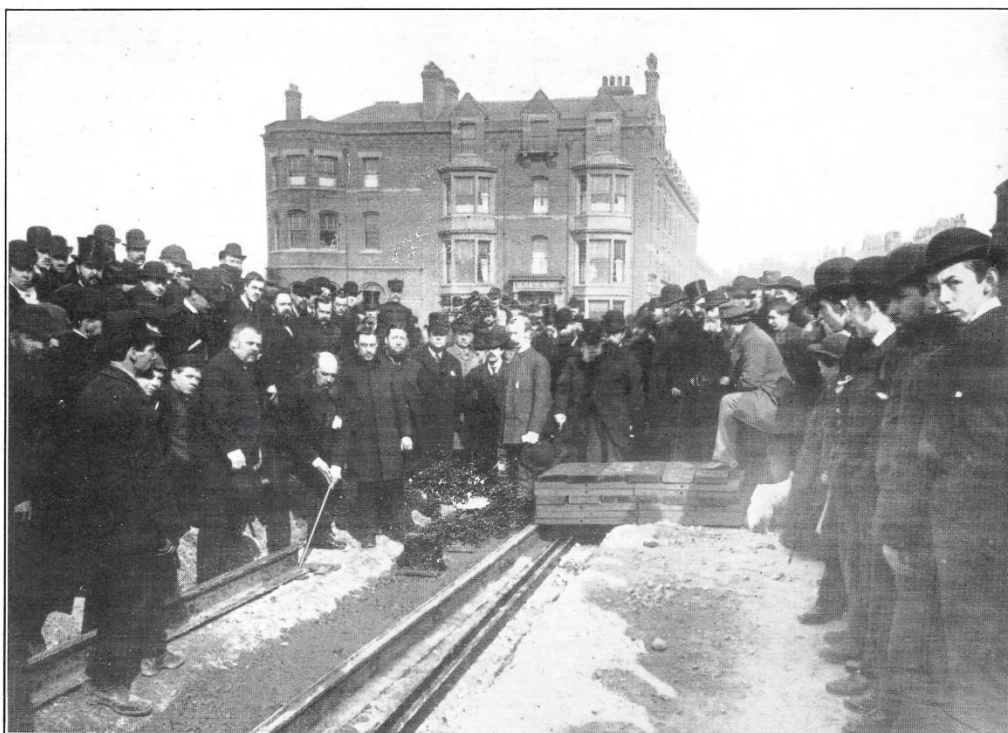
No. 114. —Placing in Position of first rail of Blackpool Corporation Tramways, 12th March, 1885. Underground Conduit System.
